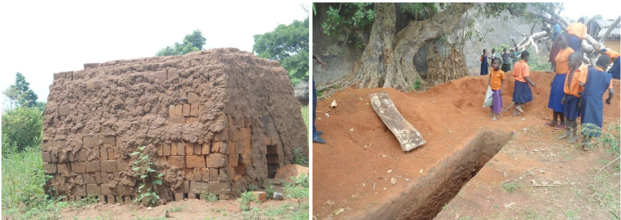
The bricks the church have baked so far (L) and a latrine they are digging for the school (R)
